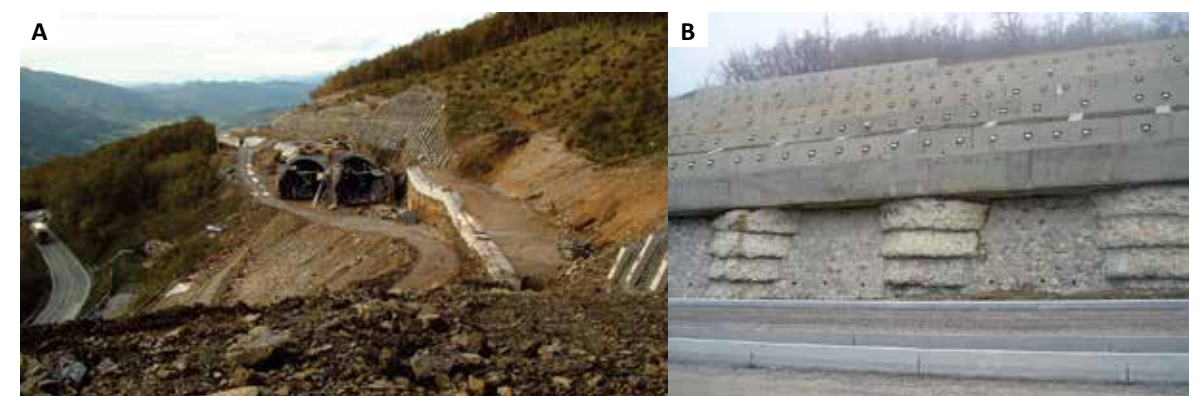
Fig. 6: A- Construction of cut and cover tunnel Rebrnice I. B- Shafts used as a retaining structure near SOR (Lozice) landslide.
