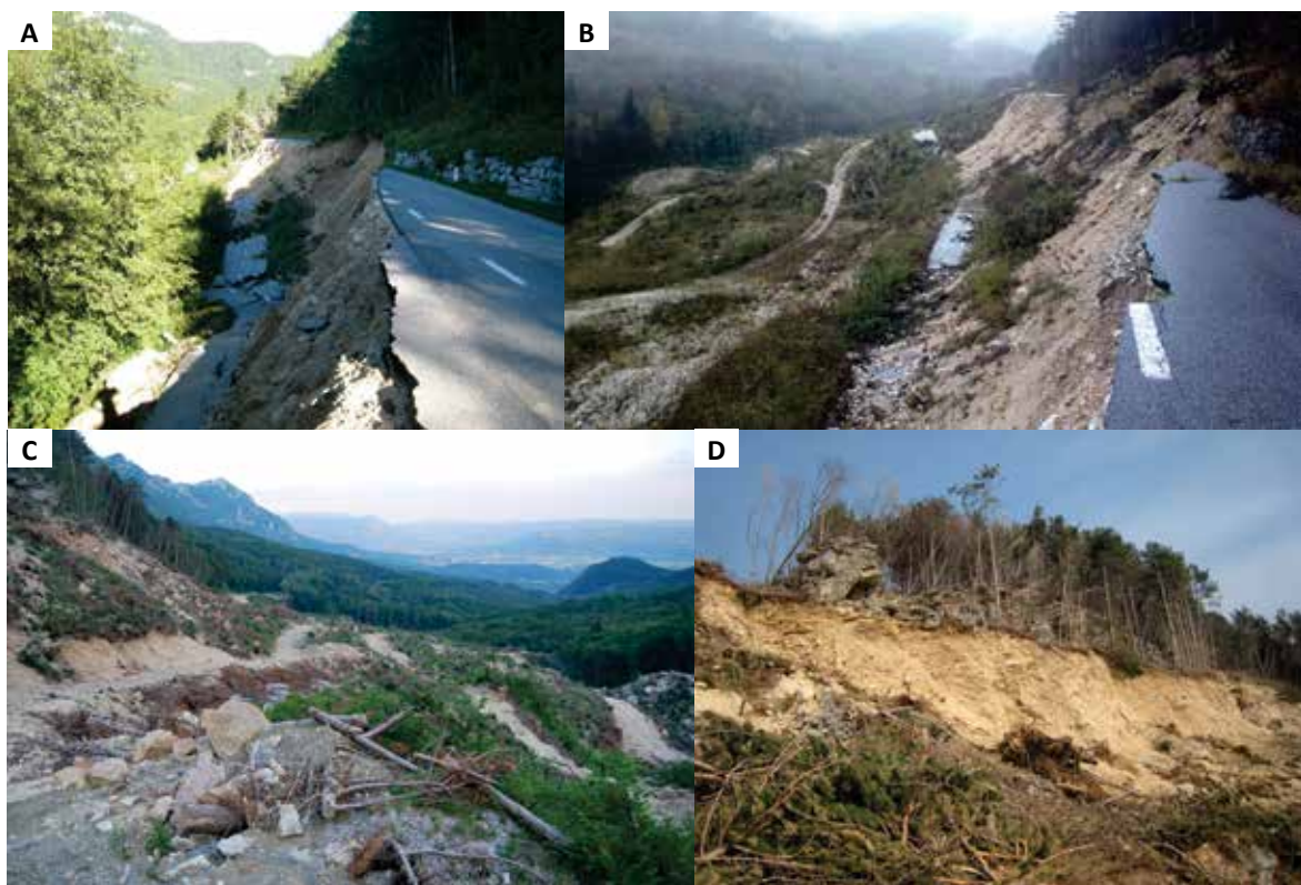
Fig. 7: Landslide Stogovce A, B- a view towards north on the destroyed road; C- The view of Stogovce landslide, view towards south; D- The main scarp. Carbonate breccia overlies carbonate scree.
