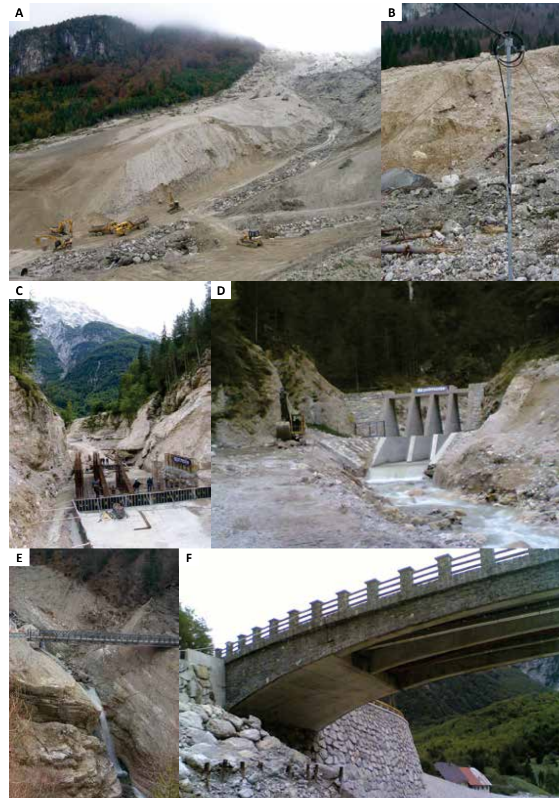
Fig. 30: Extensive remediation works: A- disposal of debris flow material; B- Early warning system; C and D- debris flow breaker during and after construction; E- two damaged roads were replaced by a temporary construction (prefabricated steel bridge); F- the new bridge.
